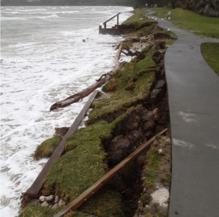
Figure 1: Snells Beach seawall and walkway damage incurred over successive 2023 coastal storm events
