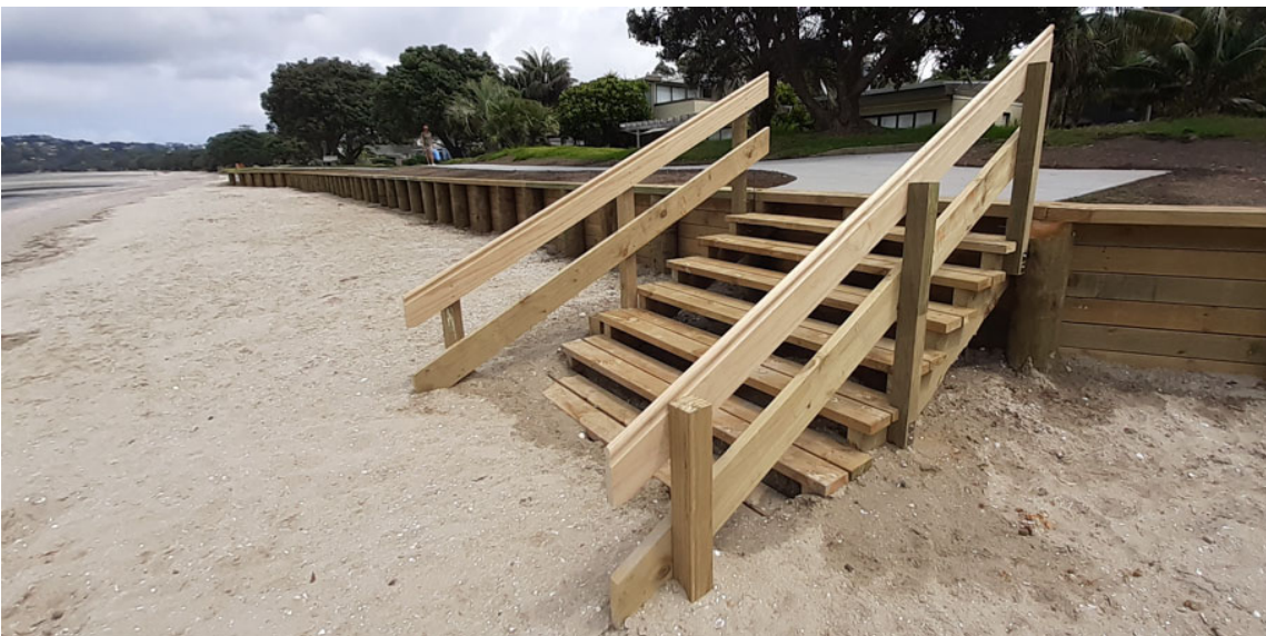
Figure 2: Completed renewal with realigned timber retaining wall and integrated beach accessways. Completed December 2023
