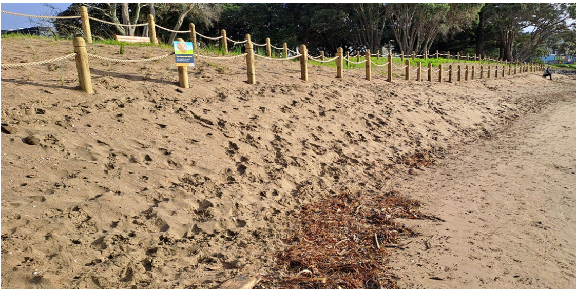
Figure 8: Browns Bay foreshore remediation including removal of legacy rock and rebuild of appropriately designed rock revetment (south of image) and naturalisation of 70m stretch including reprofiling and replanting. Stage 1 completed June 2024.
