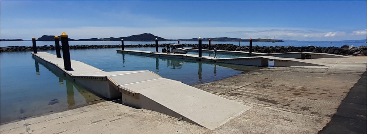
Figure 5: Pile, Pontoon and boat ramp renewal at Kawakawa Bay Boat Club, completed in December 2023
