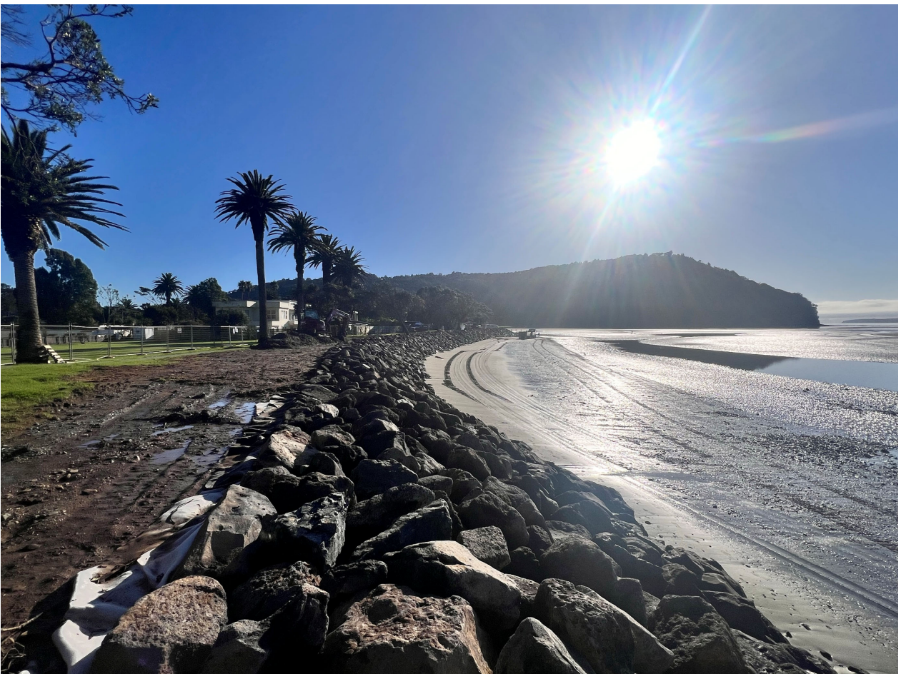
Figure 6: Re-design and reconstruction of legacy rock rip-rap with formalised and consented rock revetment. Completed June 2024
