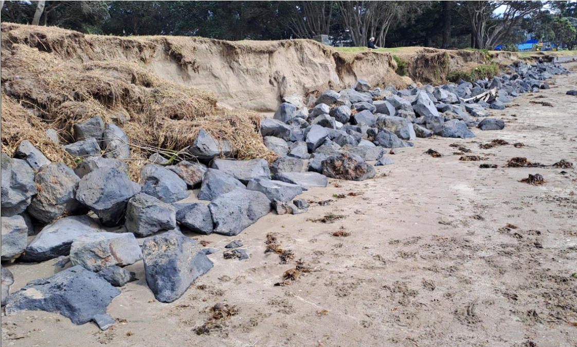
Figure 7: Significant beach erosion and exposure of legacy rock rip-rap at Browns Bay south following successive coastal storm events
