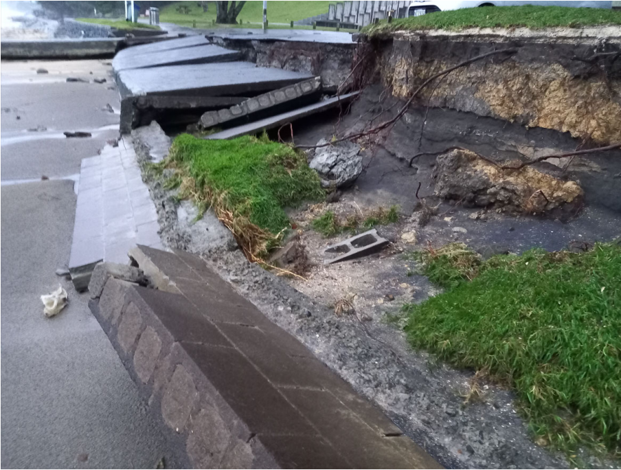
Figure 3: Murrays Bay seawall failure following Cyclone Gabrielle
